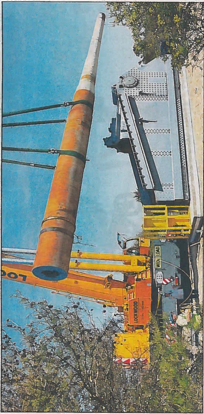
With the precision of a surgeon, a crane operator from the Virginia-based Lockwood Co., lowers the 16-inch gun onto the concrete base at Fort Miles.
