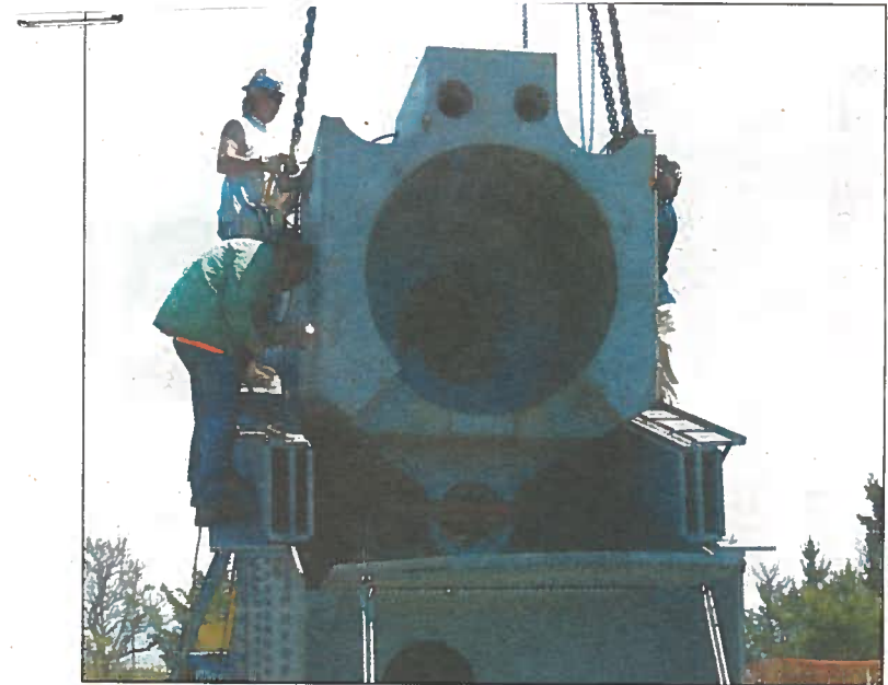
CHRIS FLOOD PHOTO A Lockwood employee welds on a bracket so the gun's yoke can be pulled into place.
